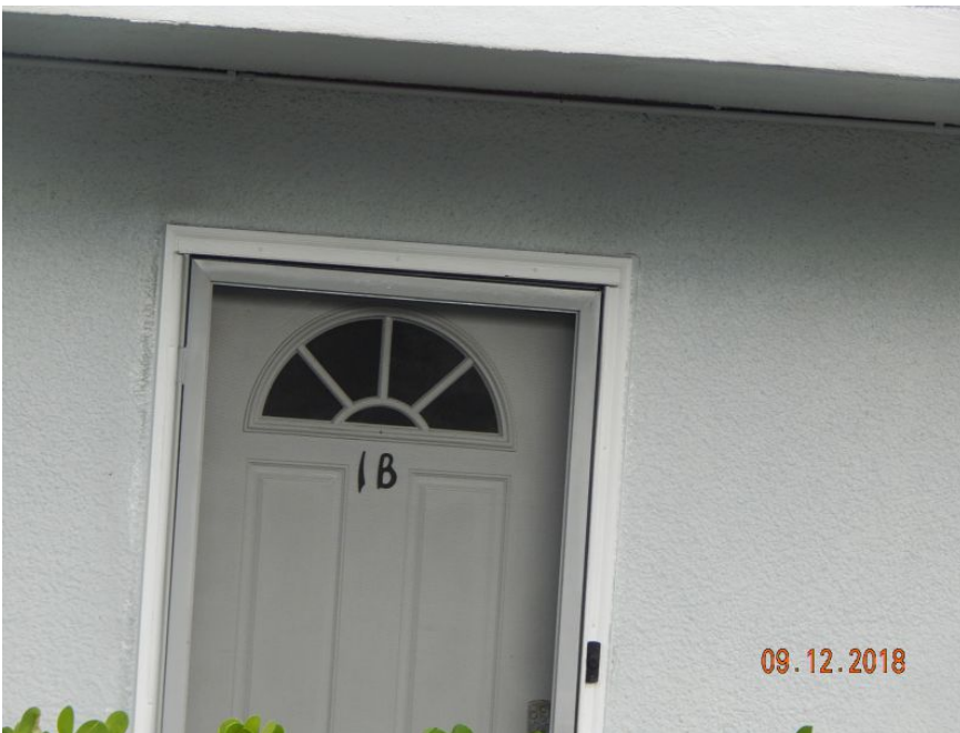
Unprotected Glazed Door
